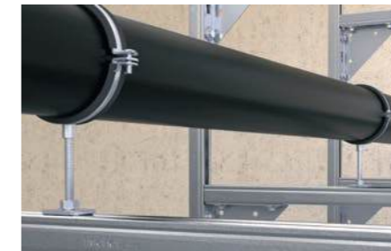
Connection on channel
