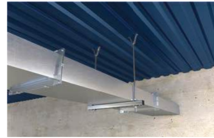
Ventilation duct on trapezoidal sheet
