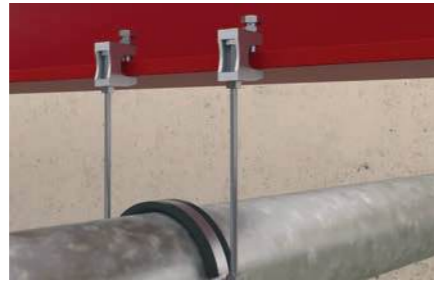
Heavy drainage pipe on beam clamp
