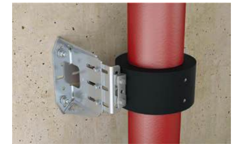
Media lines with thermal expansion
