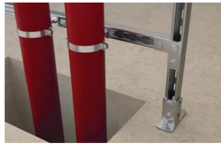
Waste water pipe
