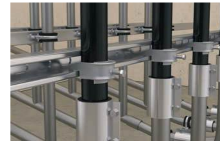
Supply lines fixed to FUS channel
