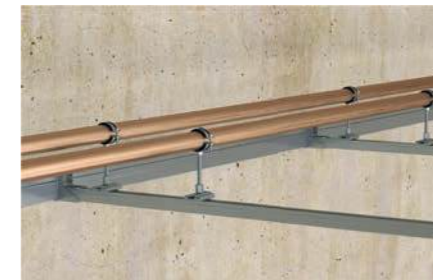
Media lines with thermal expansion
