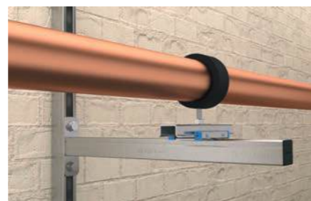
Refrigerant pipe clamp on sliding element
