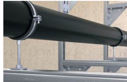
Connection on channel
