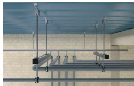
Suspended pipes on trapezoid roof
