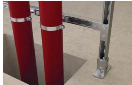
Waste water pipe
