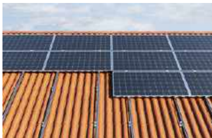
Pitched roof with tiles and landscape oriented PV panels
